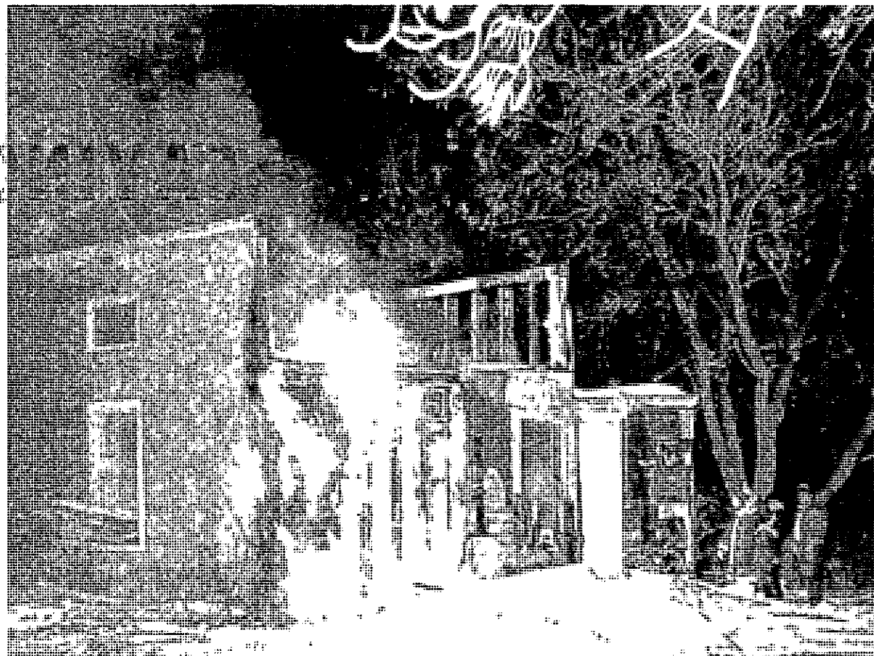
St. Johns firemen turn the tables around here as they start a fire instead of battling it. The fire department destroyed this abandoned house on S. Lansing, a structure posing a possible hazard to the area.
