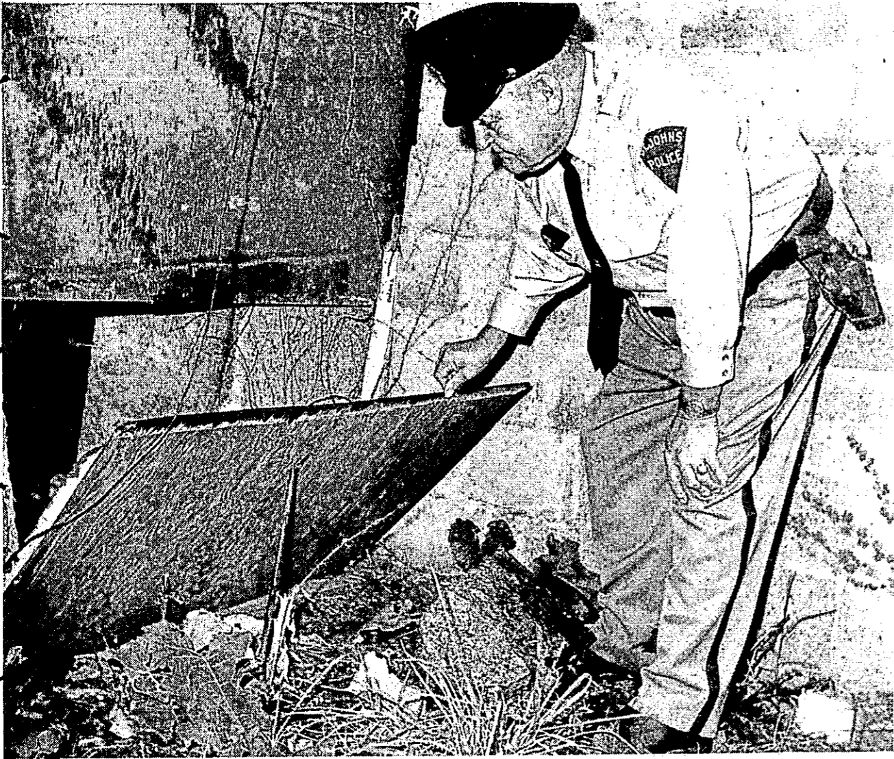
St Johns Police Everett Glazier examines the basement window at Dean's Hardware thieves pried loose Sunday night during a break-in where a large quantity of firearms and ammunition were taken. According to police, the loot which included 27 handguns, 1 shotgun, 2 rifles, 2 television sets and 52 watches totaled about $3628 in value.
