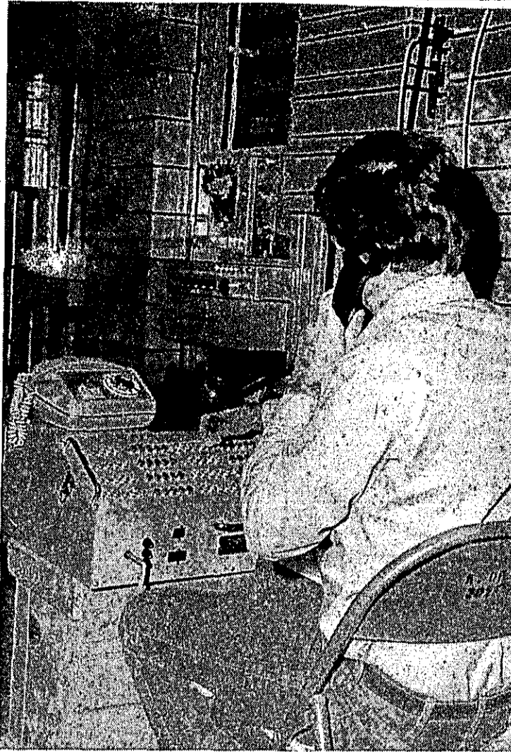
Mike Ritter, division equipment installer, tests some of the new telephone equipment at a check-out console.
