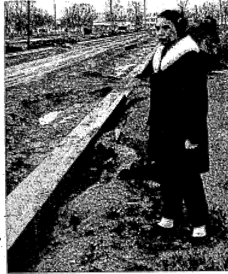
Mrs. Doyle Bancroft takes a look at Sickles Street which, though far from complete, is now passable after two months of construction that practically isolated them from the rest of the city.
