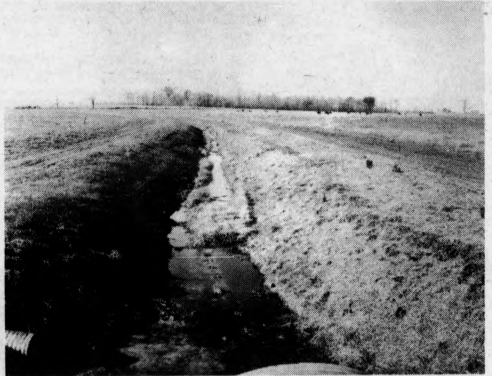
Open drain cited
